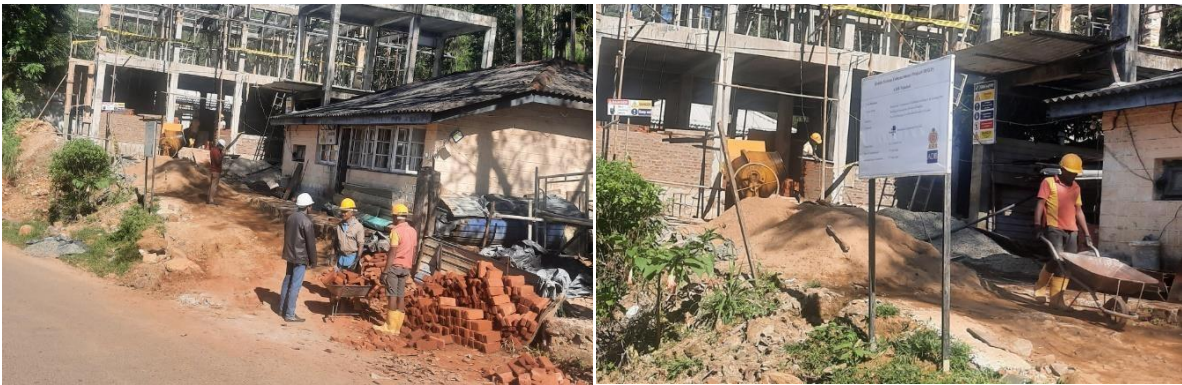
Figure **: The photographs taken by the Environmental Specialist during his site visit on February 8, 2024 – just a week before the fatal accident occurred. It is noted here that the workers were wearing appropriate PPE (hard hats, gloves and boots). However, why the workers did not wear the PPE on the day of the fatal accident is not clear.
