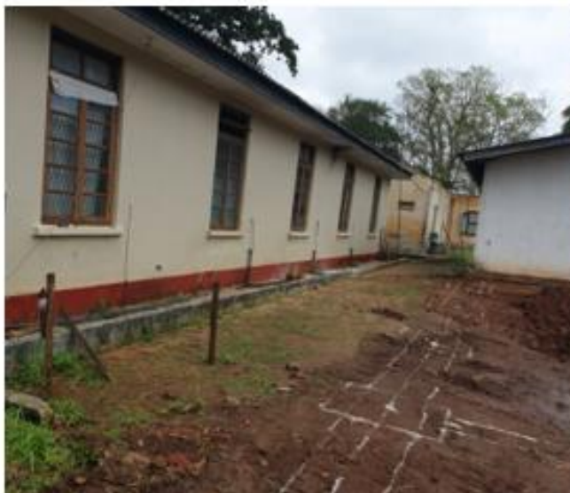
Koonwewa PMCU: Construction has commenced without erecting any dust/noise barriers
