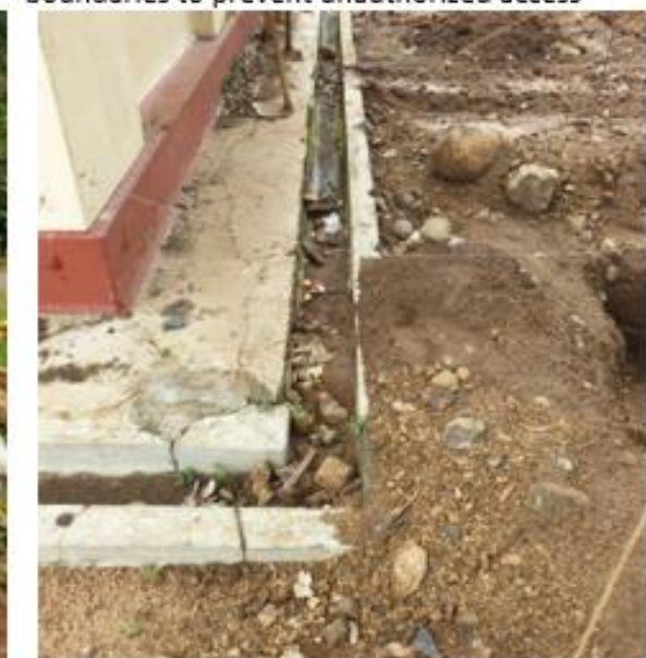
Tittagonewa PMCU: Existing drains are blocked. No dust/noise barriers
