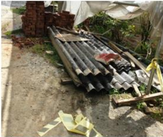
Pundalu Oya PMCU: AC Sheets stacks in the site in an unsafe manner
