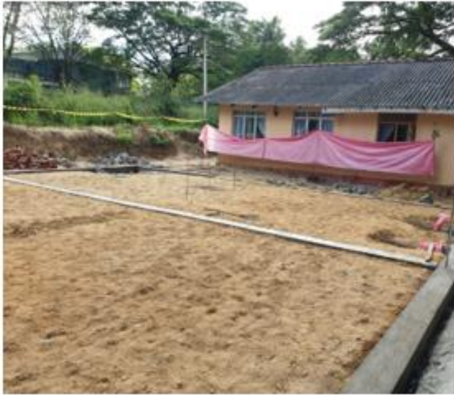
Dombagahawela PMCU: Dust barriers are not properly erected. Slopes of the access road needs strengthening.
