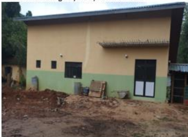
Negampaha DHC: Dust/Noise barriers needed to cover the ETU of the hospital
