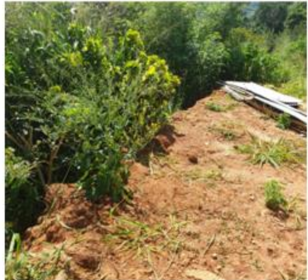
Madulkele DHB: The slope towards Galagedara Road is very unstable and needs a retaining wall
