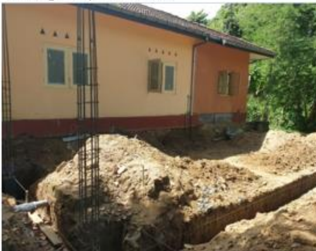
Deliwa PMCU: No proper dust/noise barriers erected in the site.
