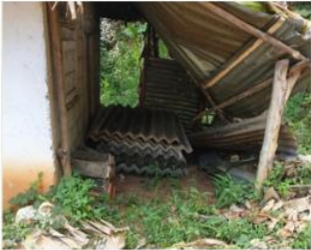
Hataraliyedda DHC: AC sheets being stored under cover, but without proper cover with polyethene
