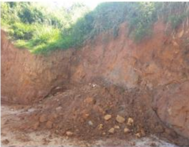
Dolosbage DHC: Unstable slopes, which need retaining walls; The slopes are unstable and water seeps through the cut slopes
