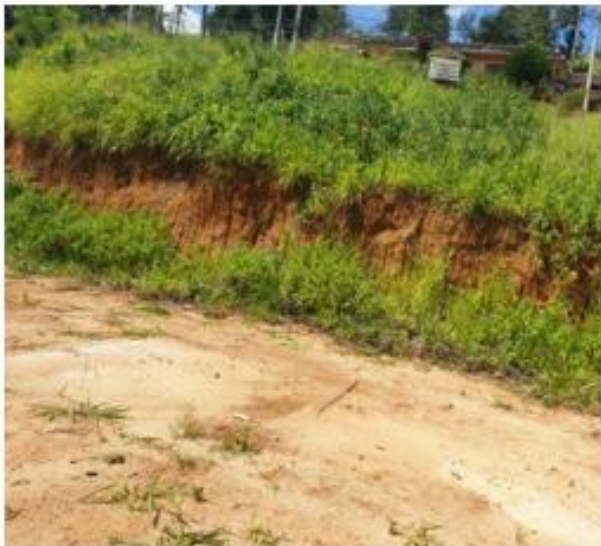
Madulkele DHB: The slope toward the hospital end needs a retaining wall. Slopes are not stable.
