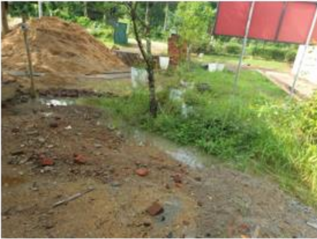
Ambagahawewa PMCU: Water logging areas within the site which need filling
