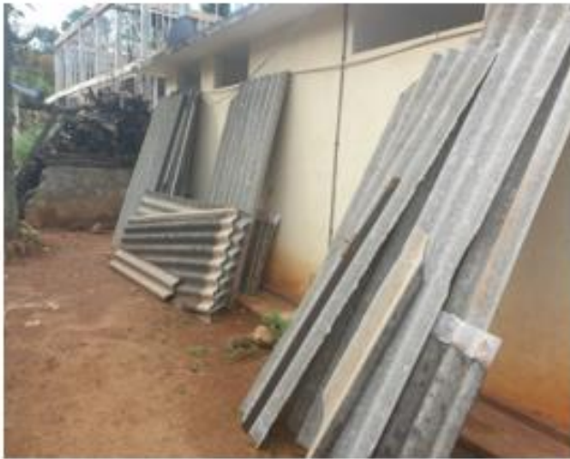
Deltota DHB: Asbestos and demolition debris at site
