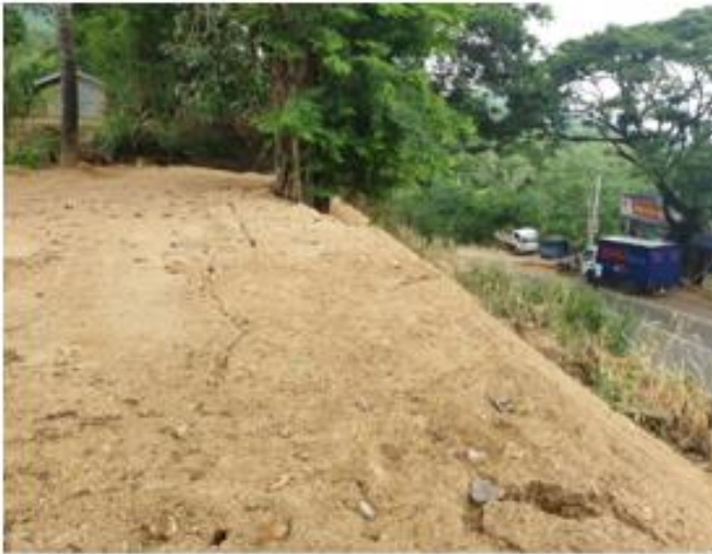
Meegahakiula DHB: Slopes that need to be stabilized and strengthened
