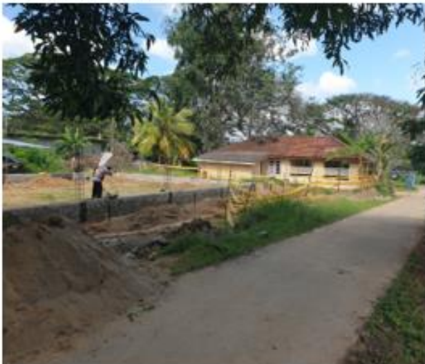
Dambagalla PMCU: Proper demarcation of the site boundaries; Sand being unloaded obstructing the access road. No dust barriers.
