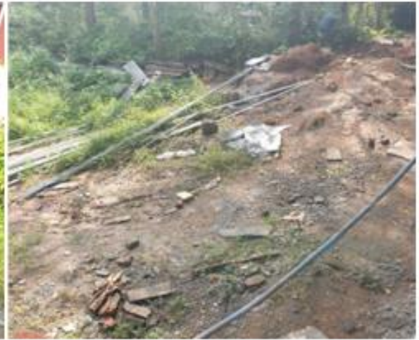
Ambagahawewa PMCU: The site needs extensive cleaning free of any debris
