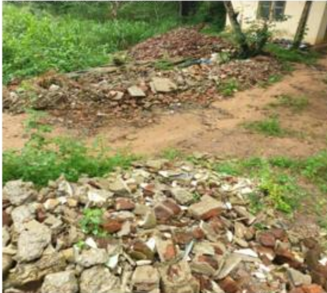
Damminna PMCU: Construction debris that needs removal from site
