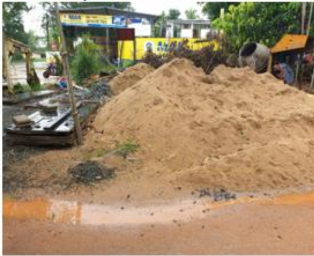
Galenbindunuwewa DHB: Sediment laden soil being washed away from the site
