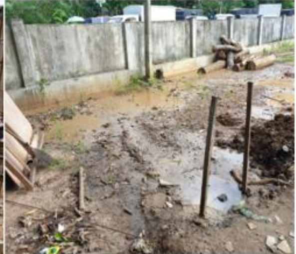
Thanamalwila DHB: Sediment laden water being discharged to road-side drains
