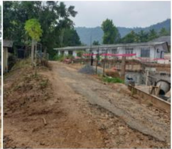
Meegahakiula DHB: Dust and noise barriers are not effective in controlling dust/noise
